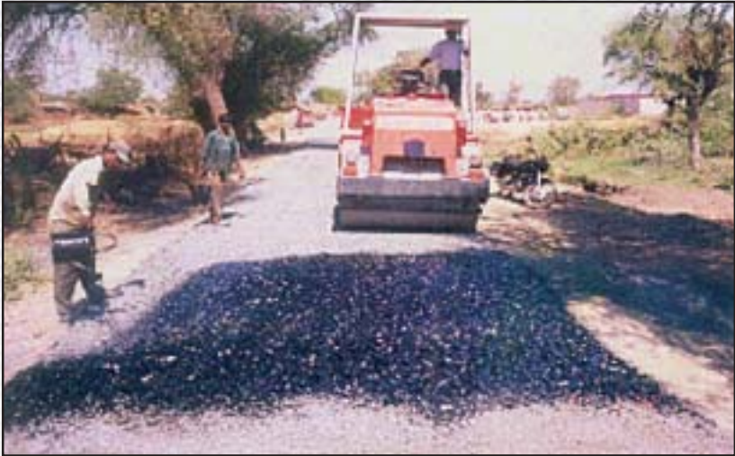
Application of binder after first coat of Surface Dressing: Pimpri Road, Orissa.
