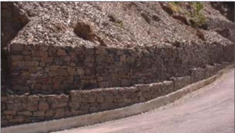
Hill side protection work and side drain: Shenal to Saunel Road, Length: 4.28 Km., Cost- 125 Lakhs, District Shimla, Himachal Pradesh.
