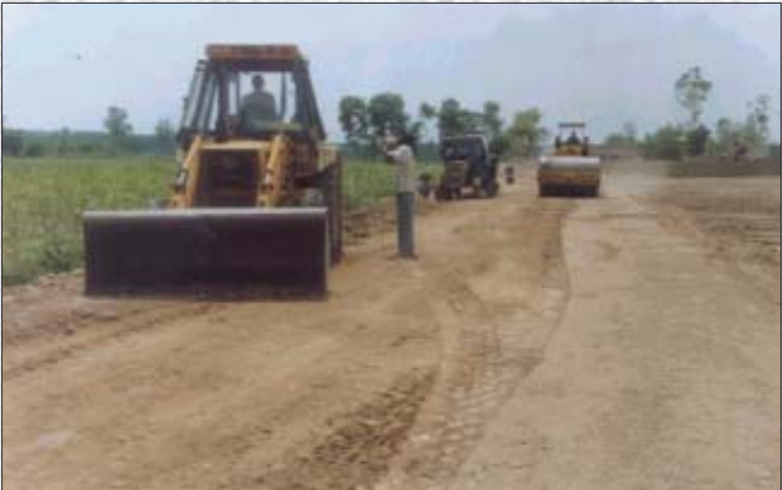
Compaction of the sub-grade soil of the road, Rampur Fakhruwal to Rampur Road, Length 2.47 Km., Cost Rs 40.55 Lakhs, Year 2001-02, District Jalandhar, Punjab.
