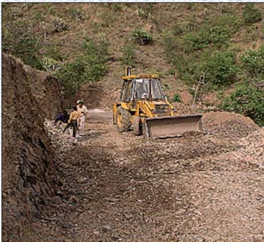
Hill side cutting for construction of formation of the road, Danughat to Kolka Road, Length:2.5 Km., Cost-62.83 Lakhs. District Solan, Himachal Pradesh.
